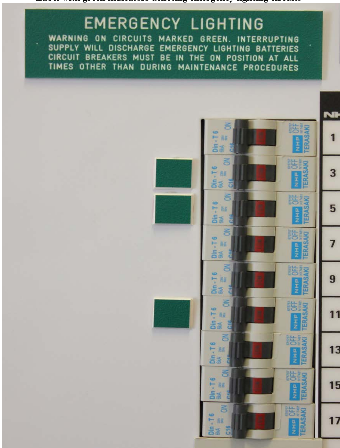
Label with green indicators denoting emergency lighting circuits
